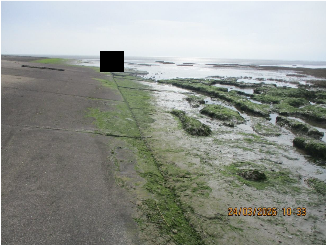
Photograph A1.7 Fragmented saltmarsh adjacent to the southwest ramp of the hoverport
